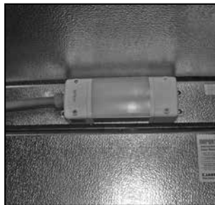
ABOVE DOOR LED LIGHT FIXTURE
